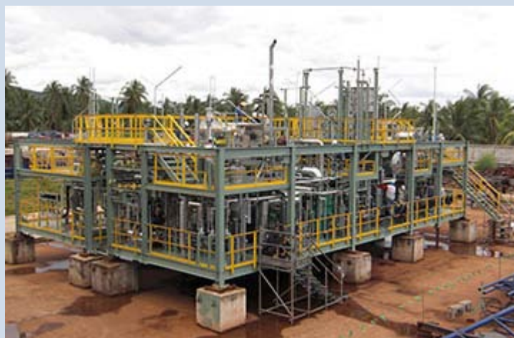
GTL skid for the Petrobras demonstration site at Fortaleza, Brazil
